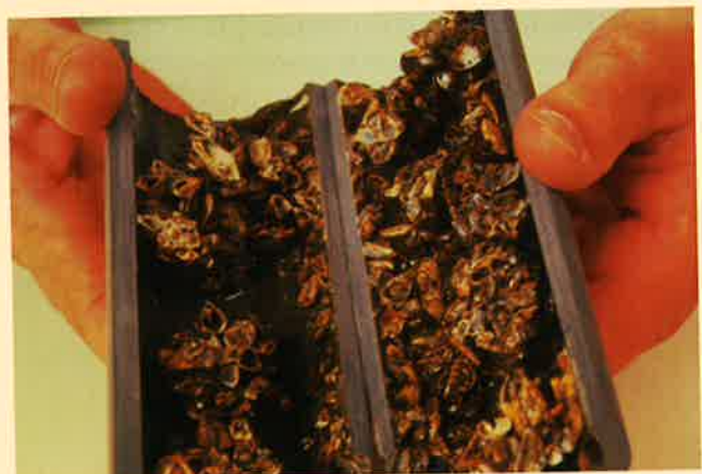
▲ Figure 6 A section through a water pipe which has been opened to reveal an interior clogged with zebra mussels, Dreissena polymorpha
